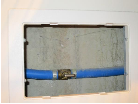
Figure 5: Suite 106 – Kitec® DCW line connecting to in-suite isolation valve.
