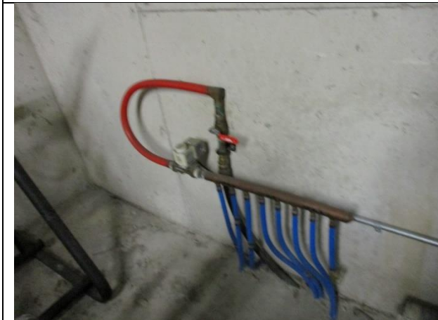
Figure 3: Kitec® piping serving trap priming manifold and Kitec® trap priming lines.
