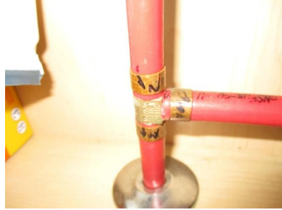
Figure 6: Suite 901: Kitec fitting within DHW distribution piping.
