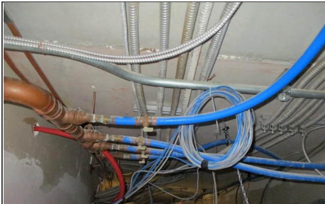
Figure 1: Typical DCW header within ceiling space in corridor.
